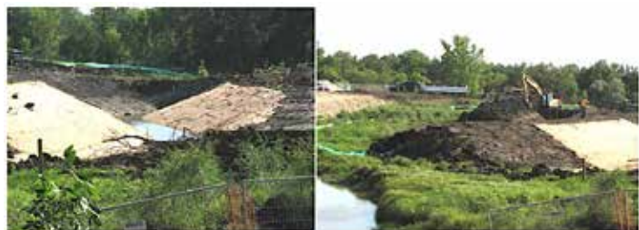
Remediation work at the IKO site, 2009. Source: Save Our Seine Newsletter. Fall Winter 2009.
